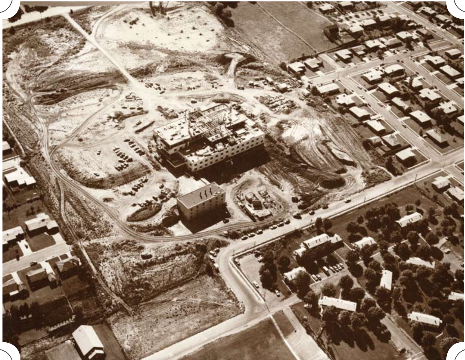
The new David O. McKay Hospital's 27-acre campus at 3939 Harrison Boulevard took shape rapidly as crews worked to meet the completion deadlines.
